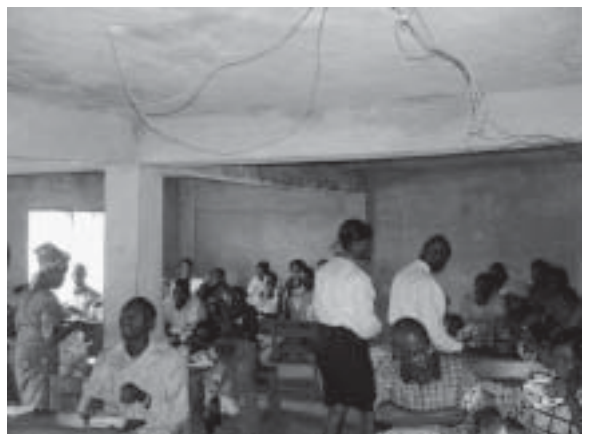
right: Electric wirings hanging from ceiling.
