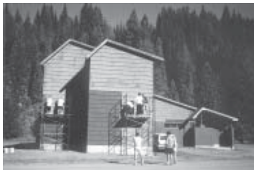
Mill Neck students on scaffolding paint a dormitory at the Shoshone Base Camp for their Servanthood Project.
